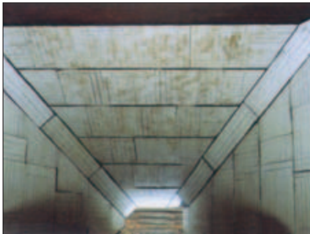
輸送機落料槽 Unloading hopper for conveyor line
